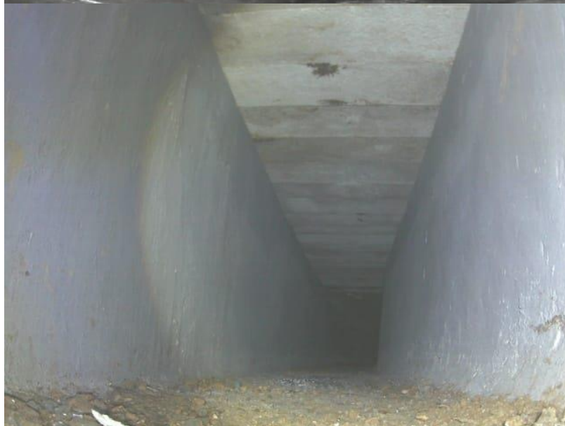
Figures 3, 4, and 5: examples of Enel canals.
